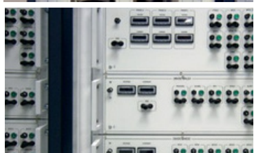
Support Center for TIGER Power racks to control the distribution of 115VAC/400Hz and 28VDC
