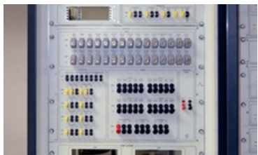
Support Center for TIGER Equipment racks with breakout and patching panels
