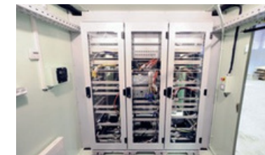
Ground control station Equipment racks inside the shelter
